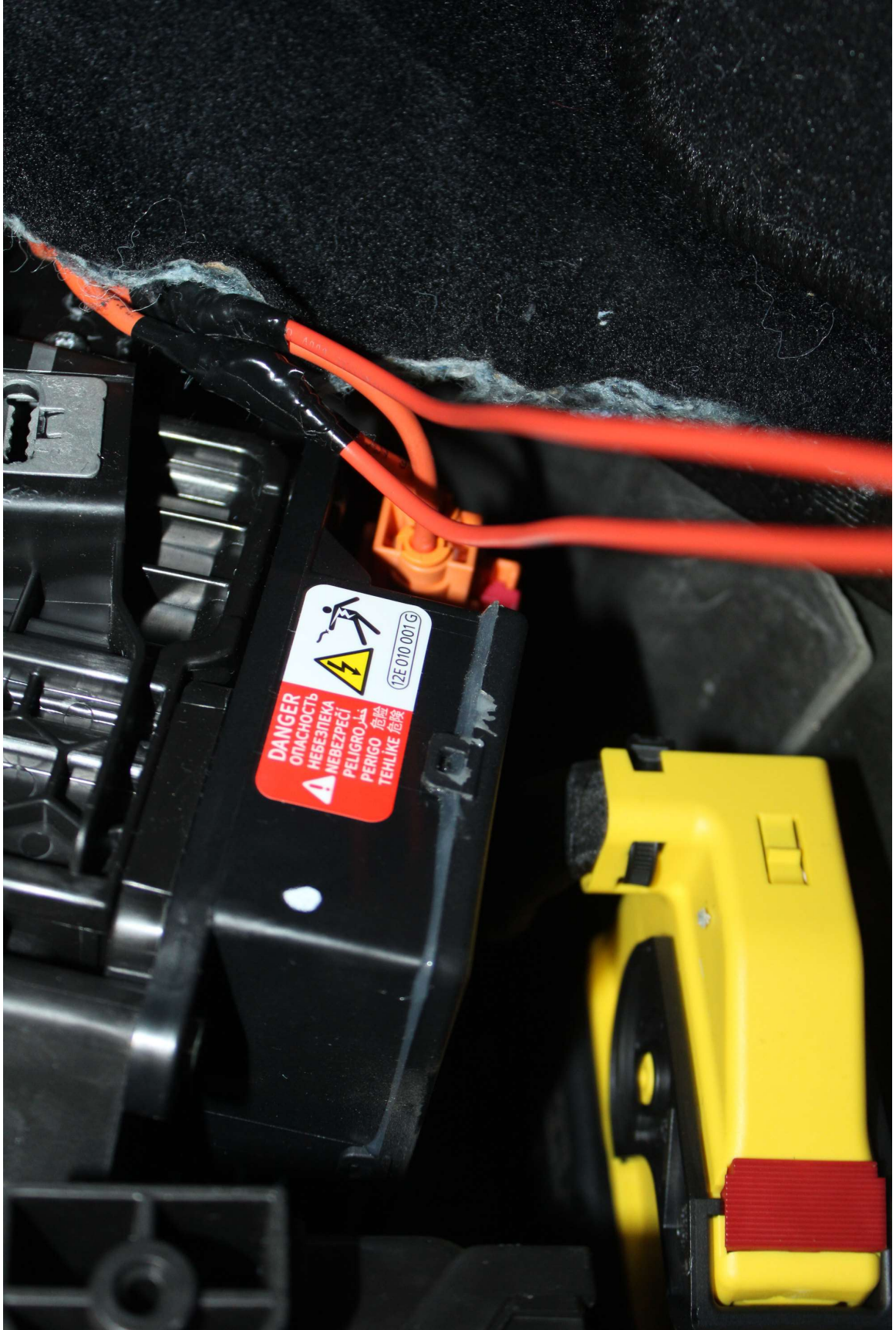
Photo No. 70. Pre-Test Voltage Monitoring Leads Attached to Electric Energy Storage System
