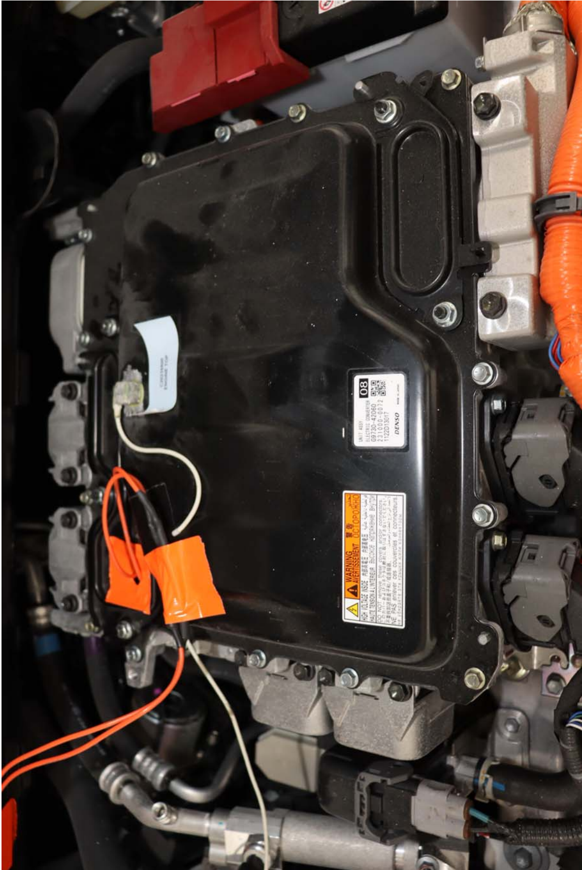
Photo No. 74. Pre-Test Voltage Monitoring Leads Exit From Outside Electric Energy Storage System
