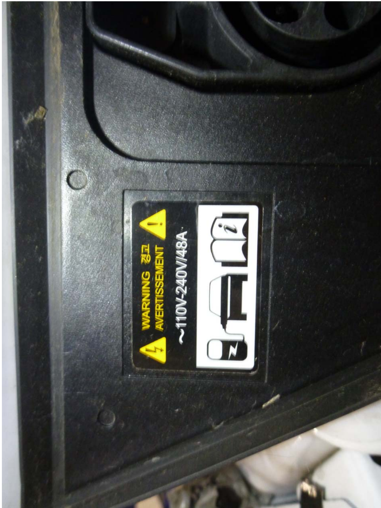
Photo No. 63. High Voltage Warning Label
