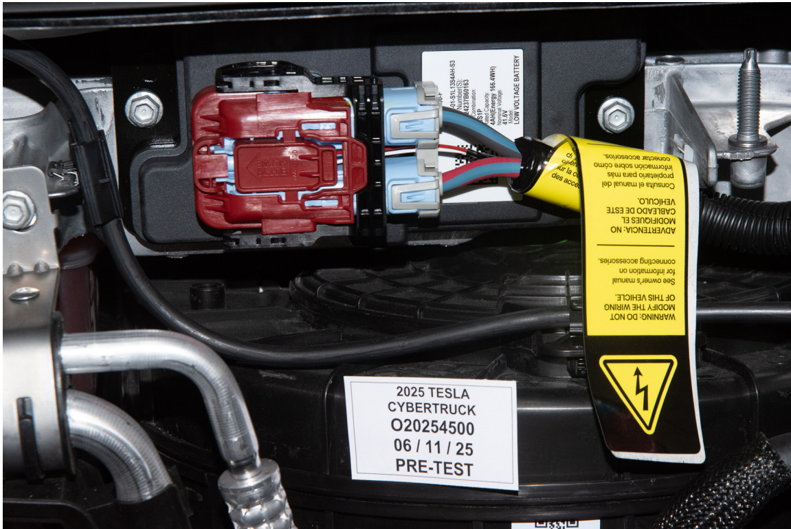
FIGURE 305-018. Pre-Impact View of High Voltage Interconnect(s)
