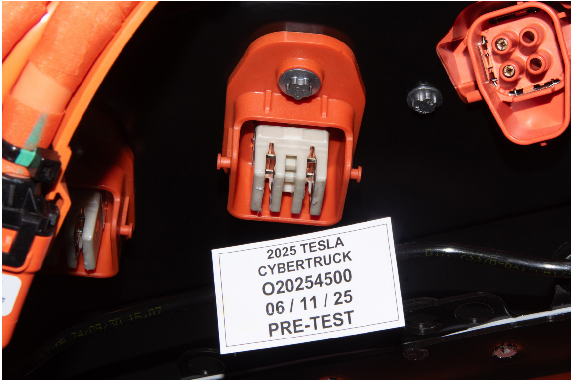
FIGURE 305-08b Manual High Voltage Service Disconnect Removed
