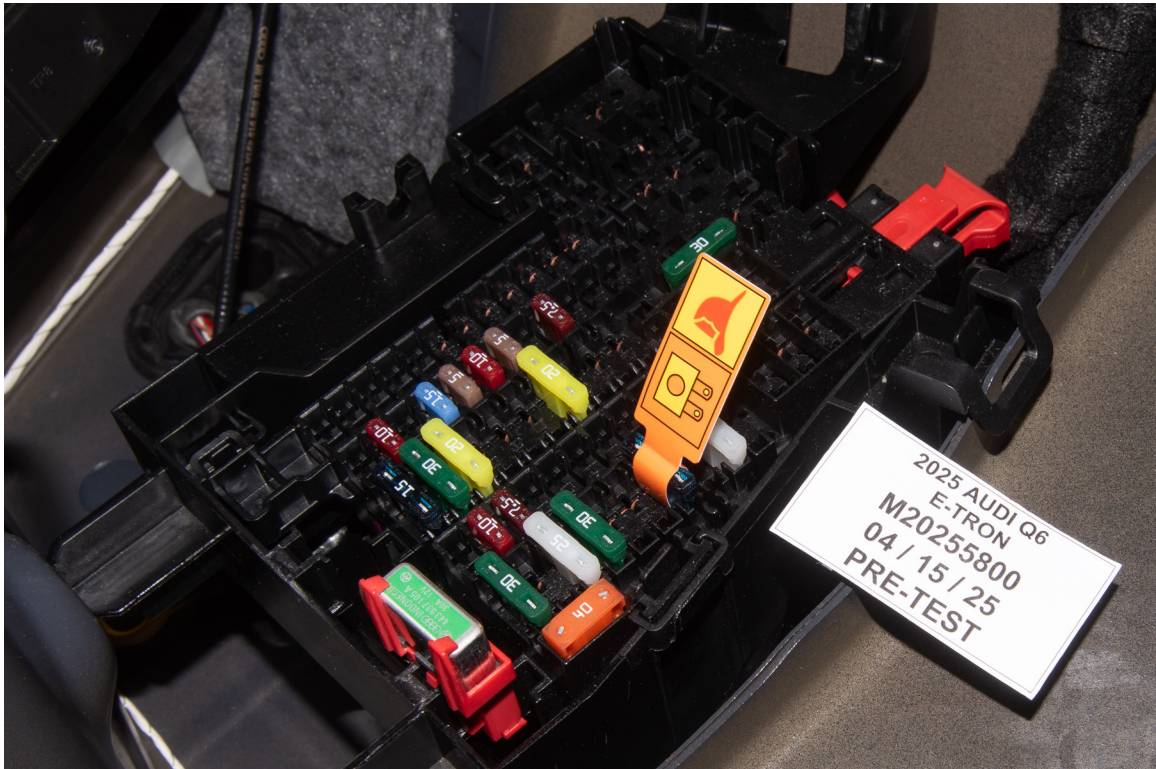
FIGURE 305-03a. First Responder Warning Label
