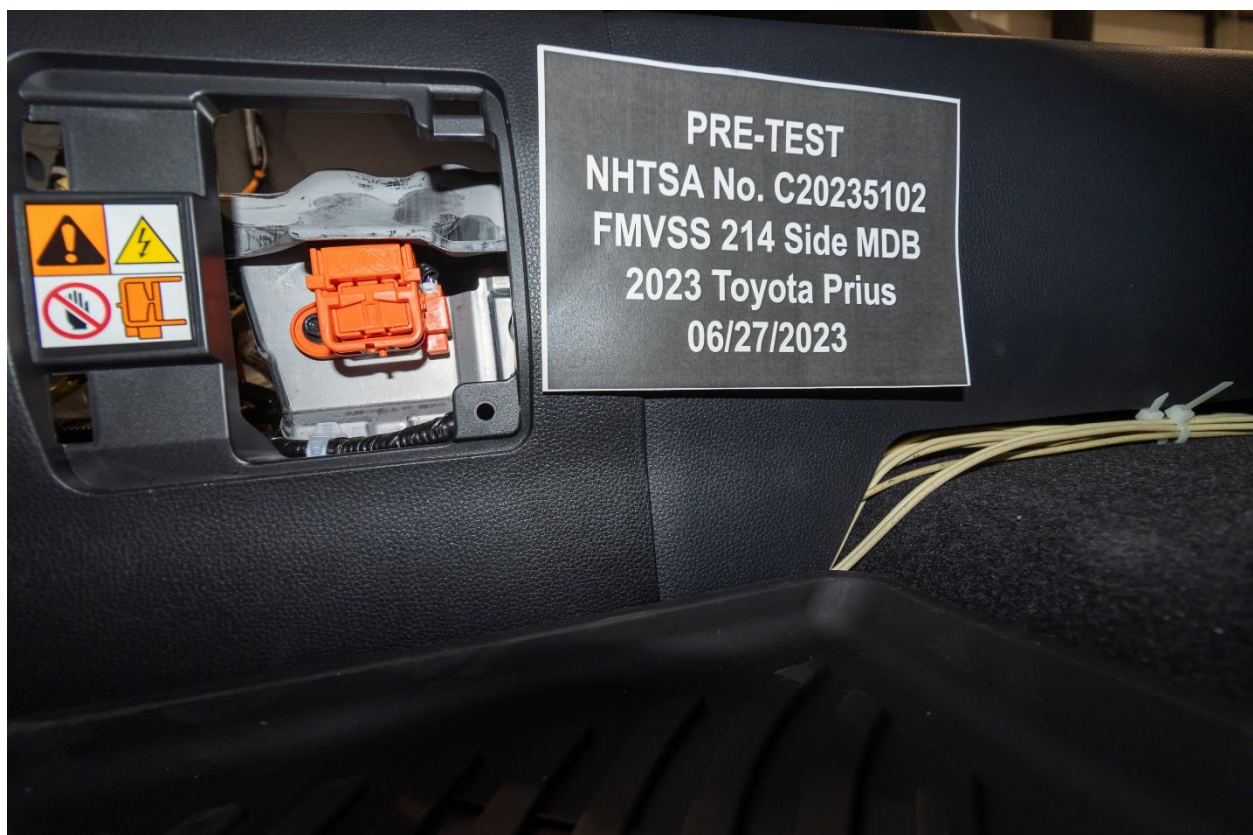
Figure 305-6: Manual High Voltage Service Disconnect in Place
