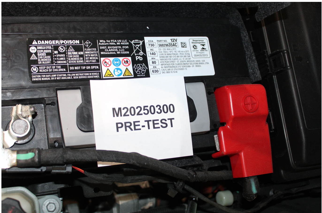
Photo No. 305-01 - Auxiliary Power Module Warning Label
