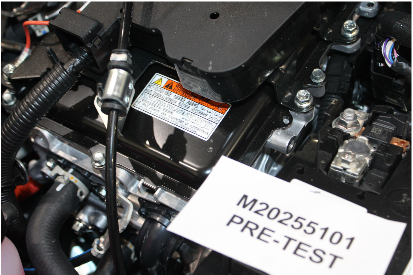
Photo No. 305-02 - Power Inverter Warning Label
