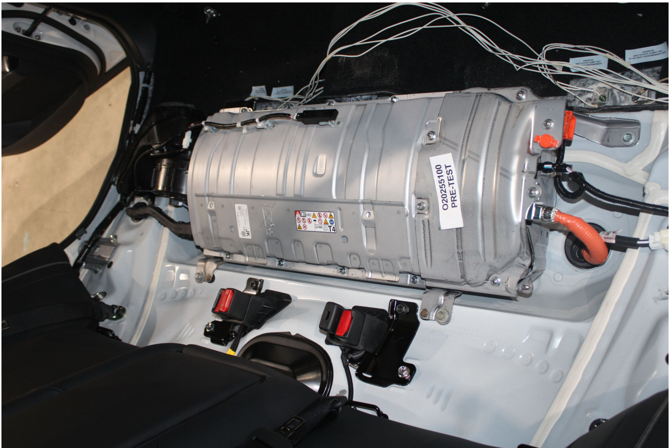
Photo No. 305-09 - Pre-Impact View of Propulsion Battery
