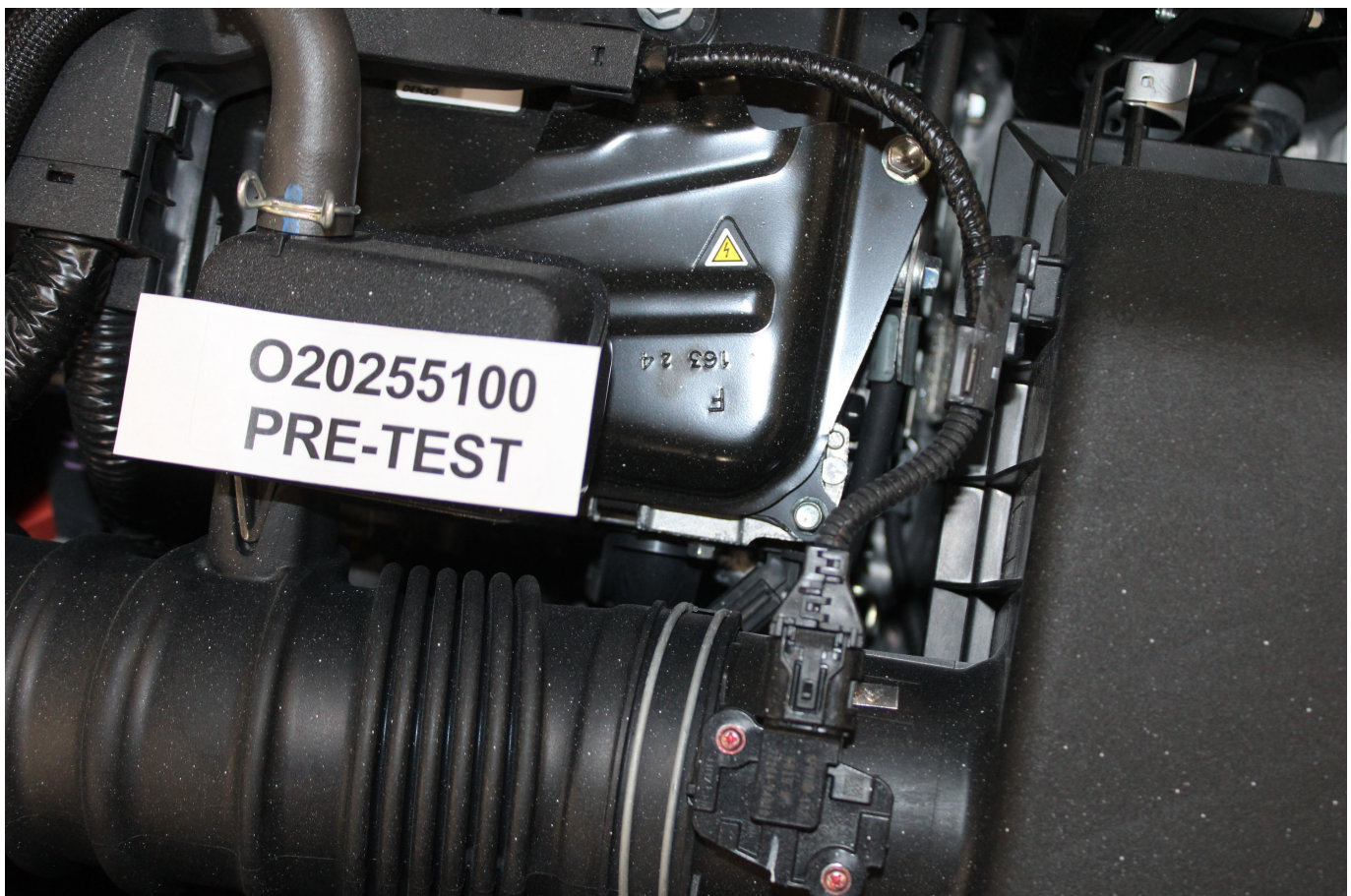
Photo No. 305-02 - Power Inverter Warning Label
