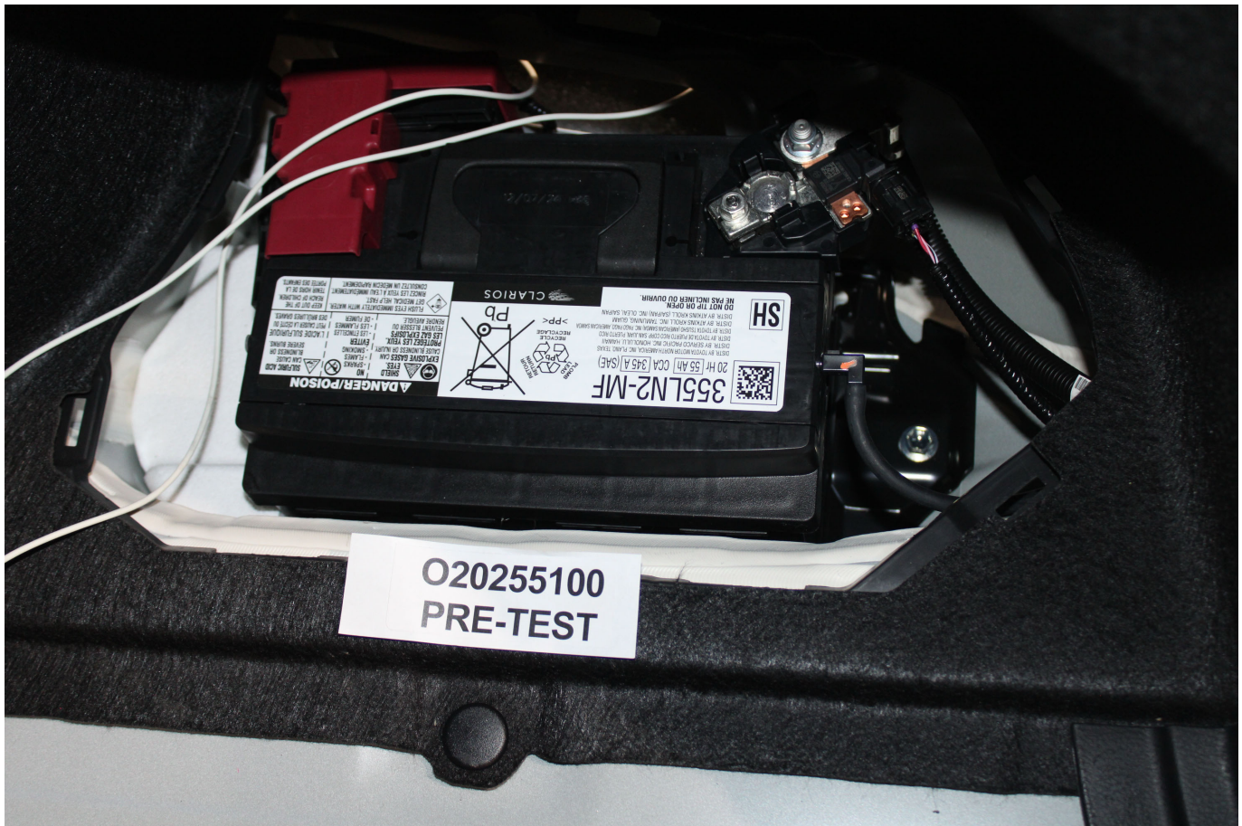
Photo No. 305-01 - Auxiliary Power Module Warning Label
