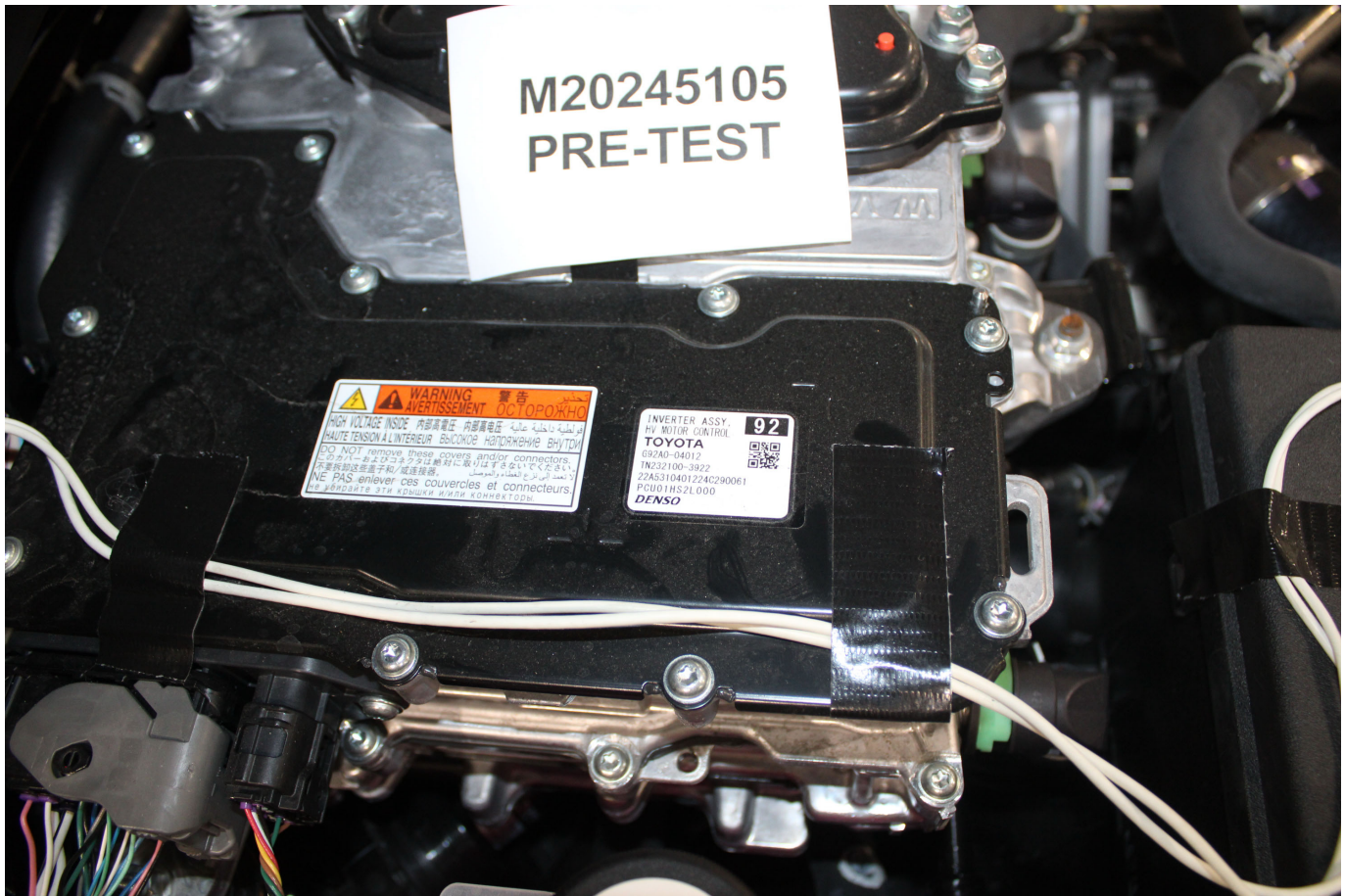
Photo No. 305-02 - Power Inverter Warning Label
