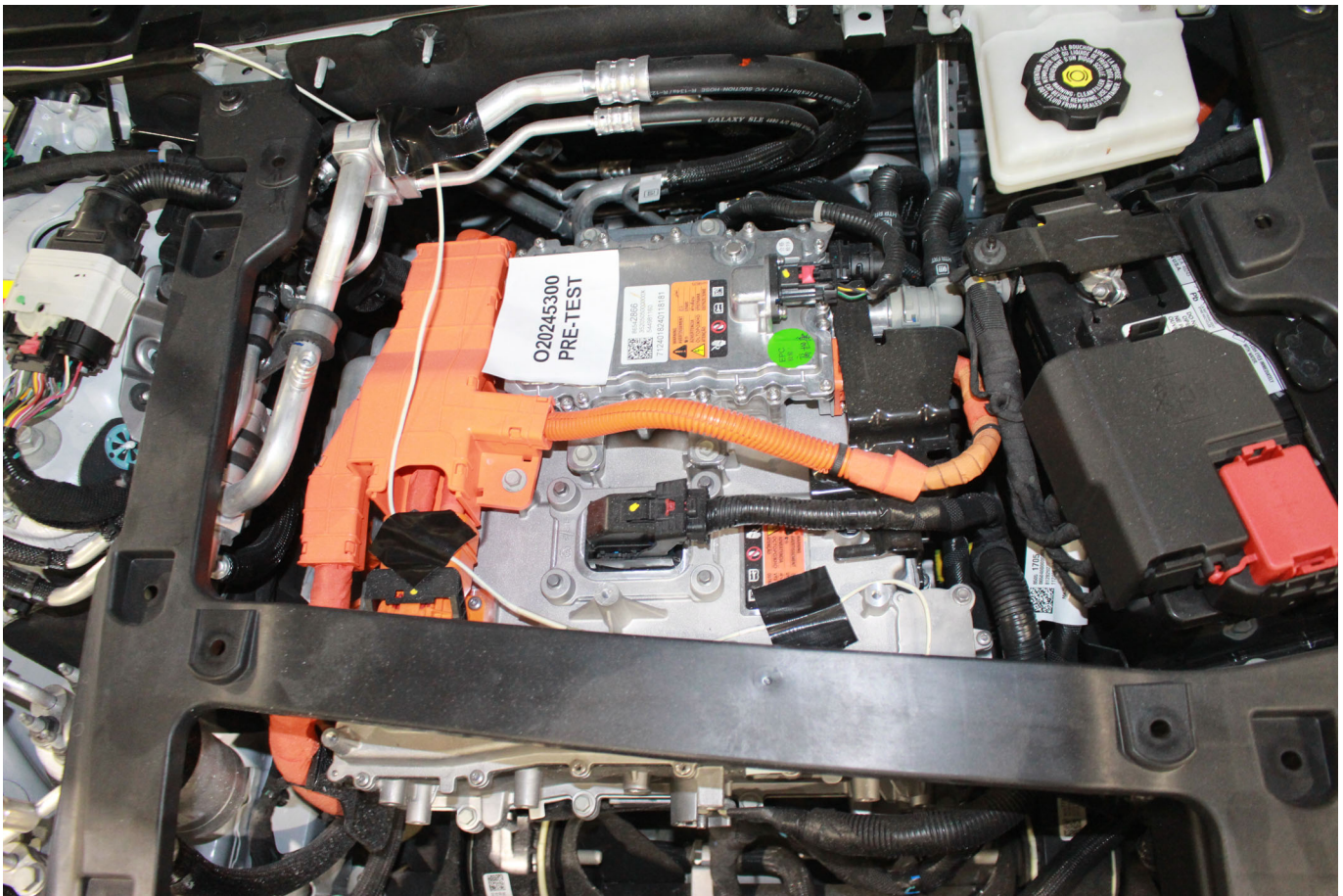
Photo No. 305-02 - Power Inverter Warning Label
