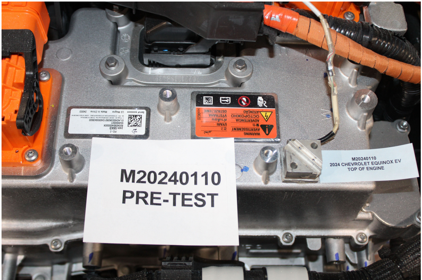
Photo No. 305-02 - Power Inverter Warning Label
