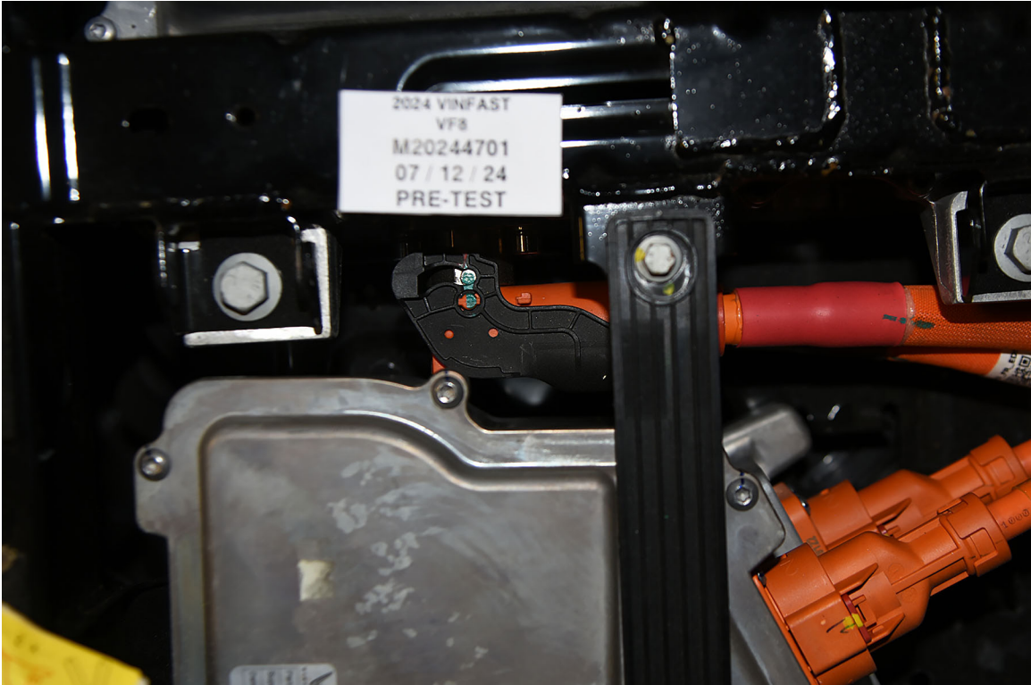
FIGURE 305-018 Pre-Impact View of High Voltage Interconnect(s)
