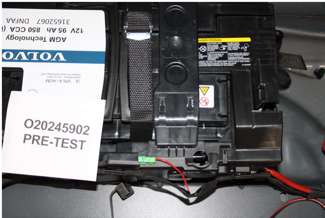
Photo No. 305-01 - Auxiliary Power Module Warning Label
