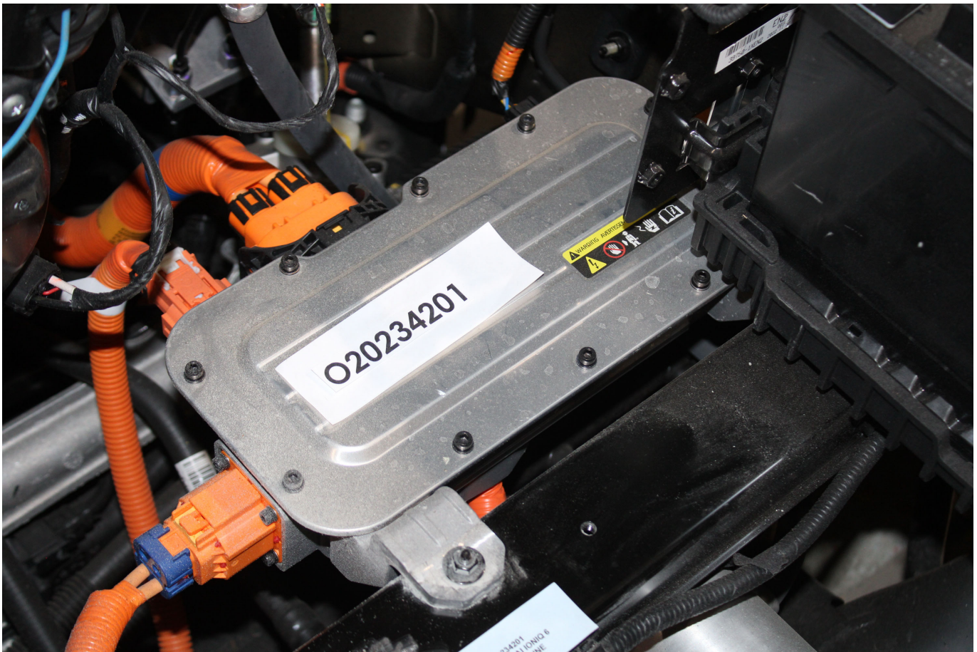
Photo No. 305-02 - Power Inverter Warning Label
