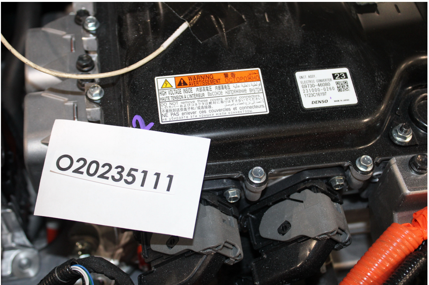
Photo No. 305-02 - Power Inverter Warning Label
