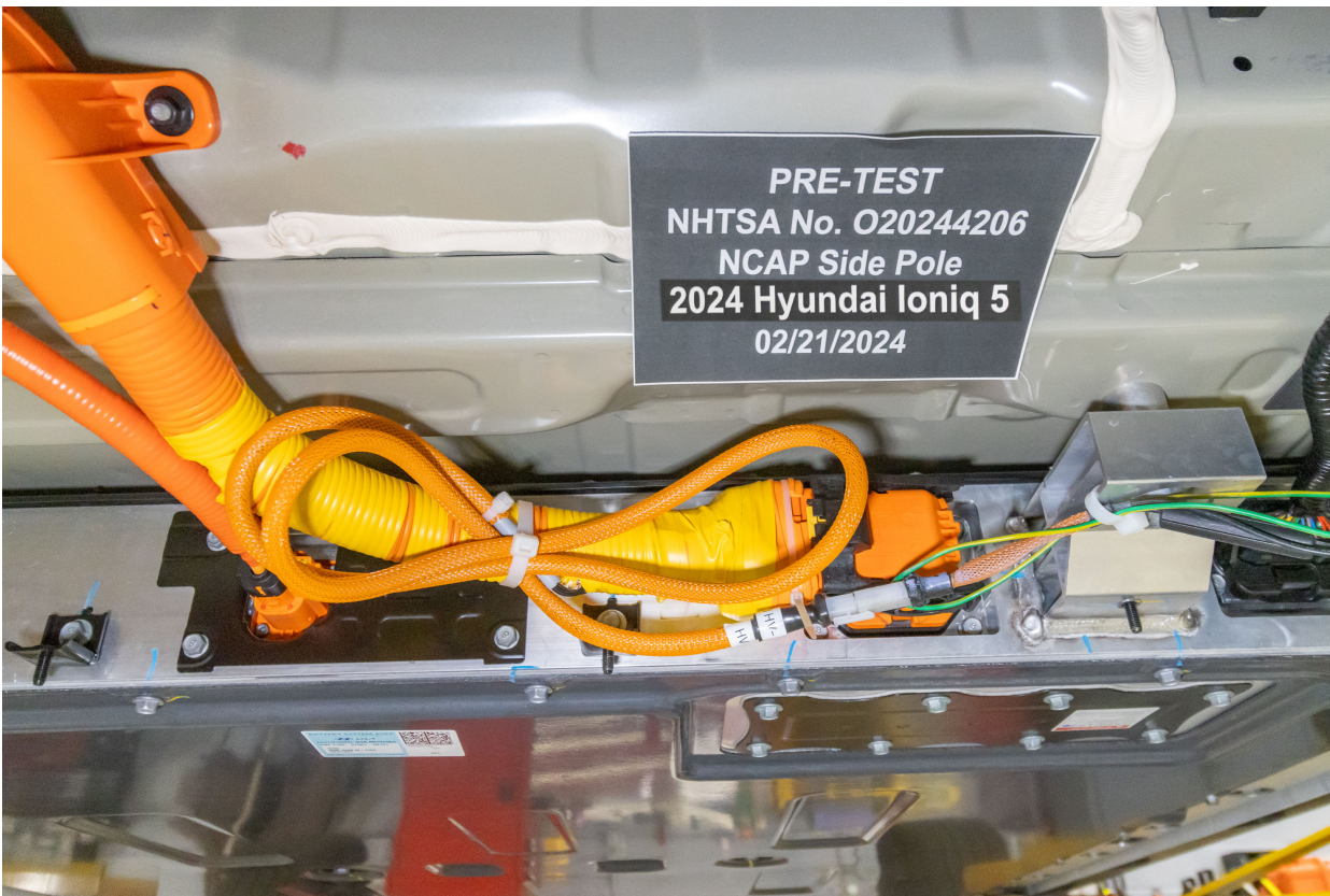
Figure 305-18: Pre-Impact View of High Voltage Interconnects
