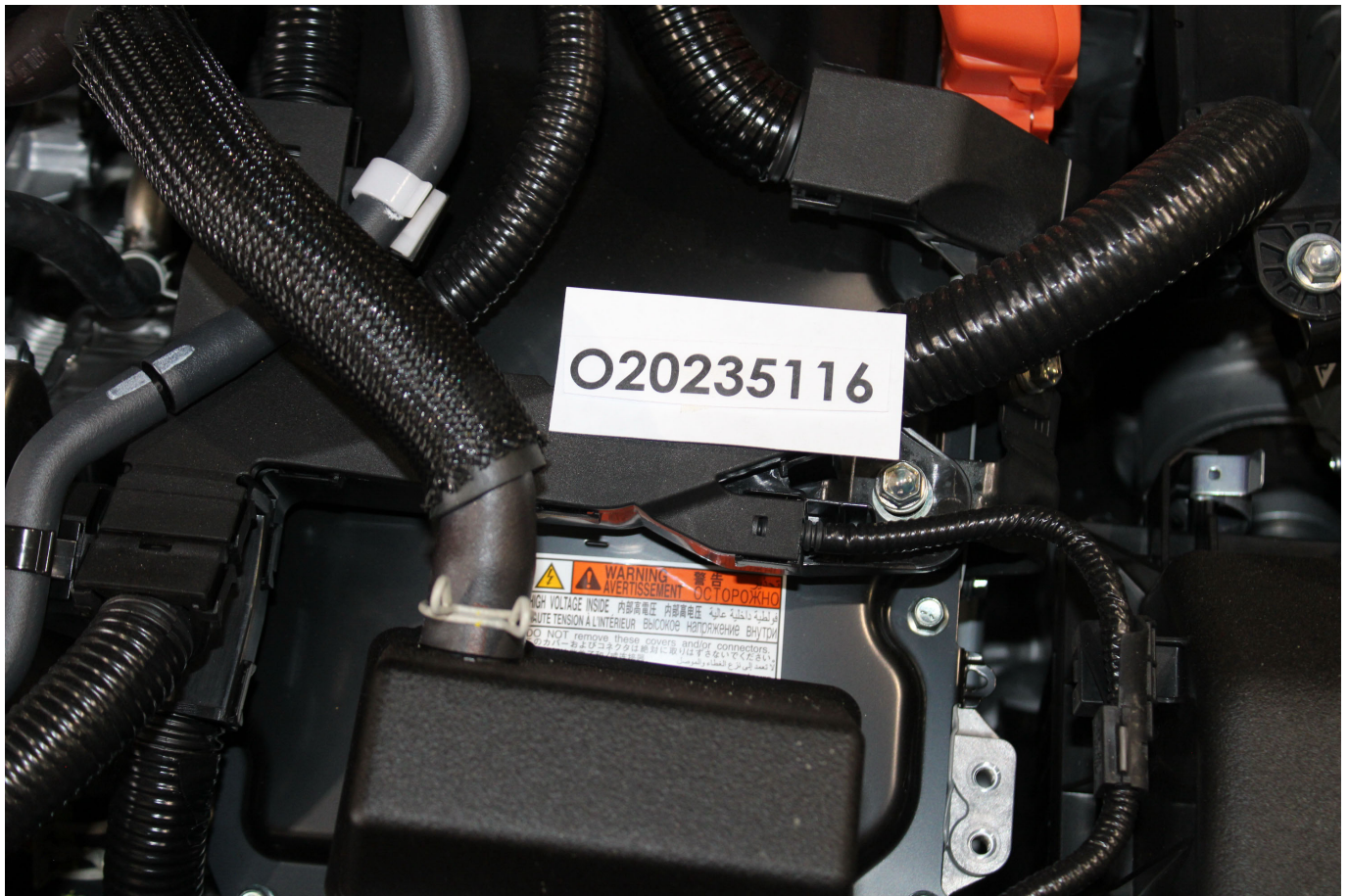
Photo No. 305-02 - Power Inverter Warning Label
