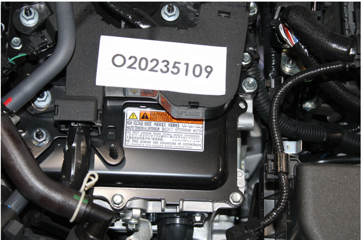
Photo No. 305-02 - Power Inverter Warning Label
