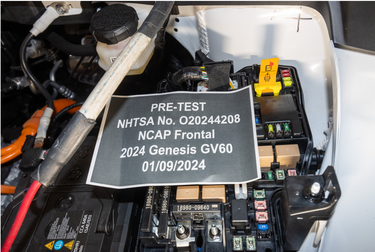
Figure 305-6: Manual High Voltage Service Disconnect in Place
