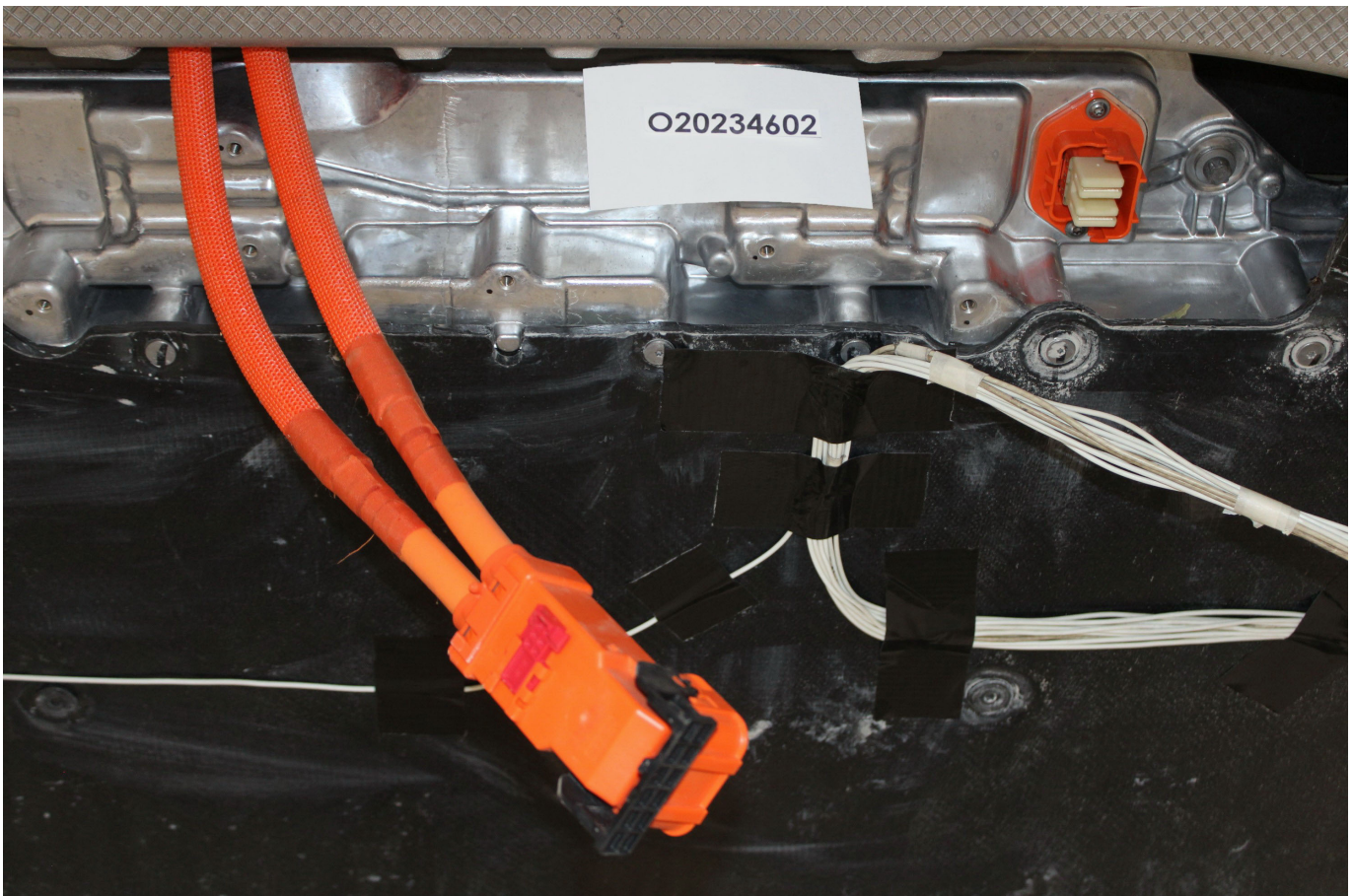
Photo No. 305-18 - Pre-Impact View of High Voltage Interconnect(s)
