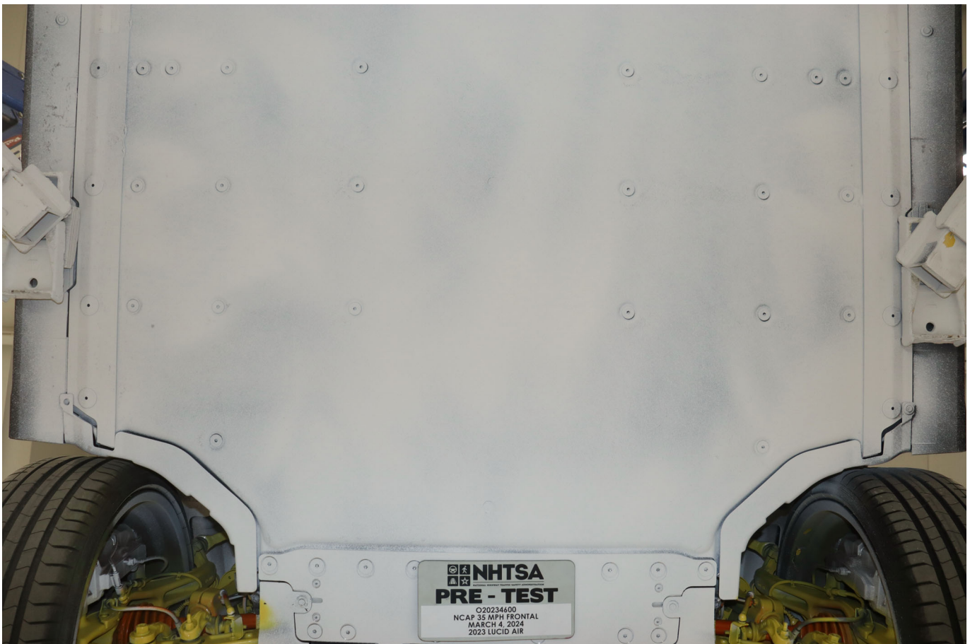
Photo No. 305-09 - Pre-Impact View of Propulsion Battery
