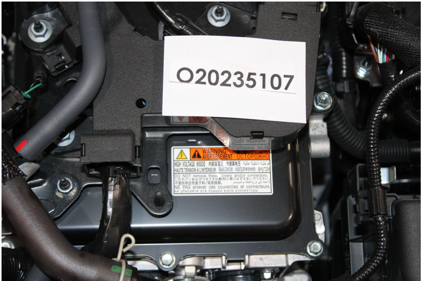
Photo No. 305-02 - Power Inverter Warning Label
