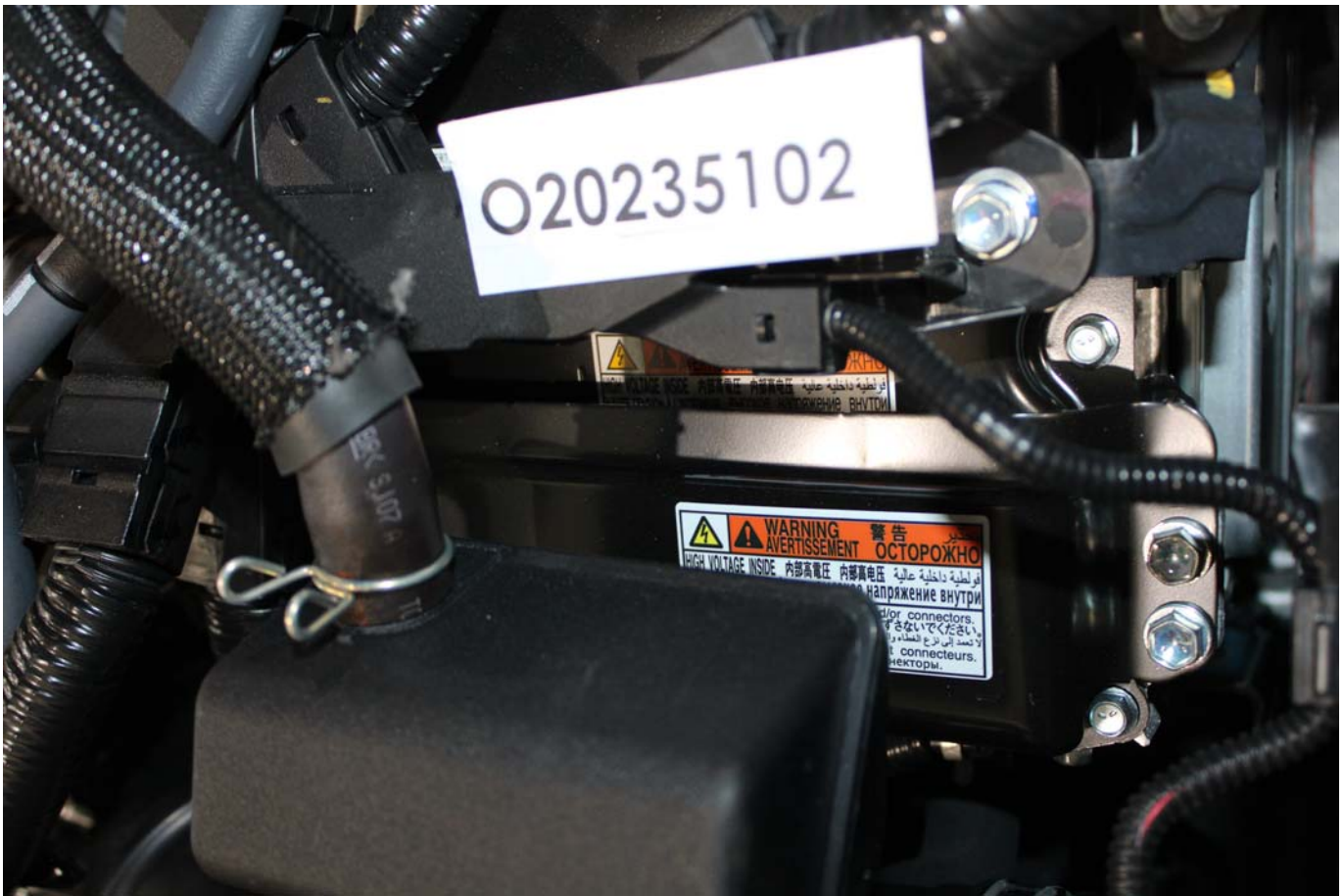
Photo No. 305-02 - Power Inverter Warning Label
