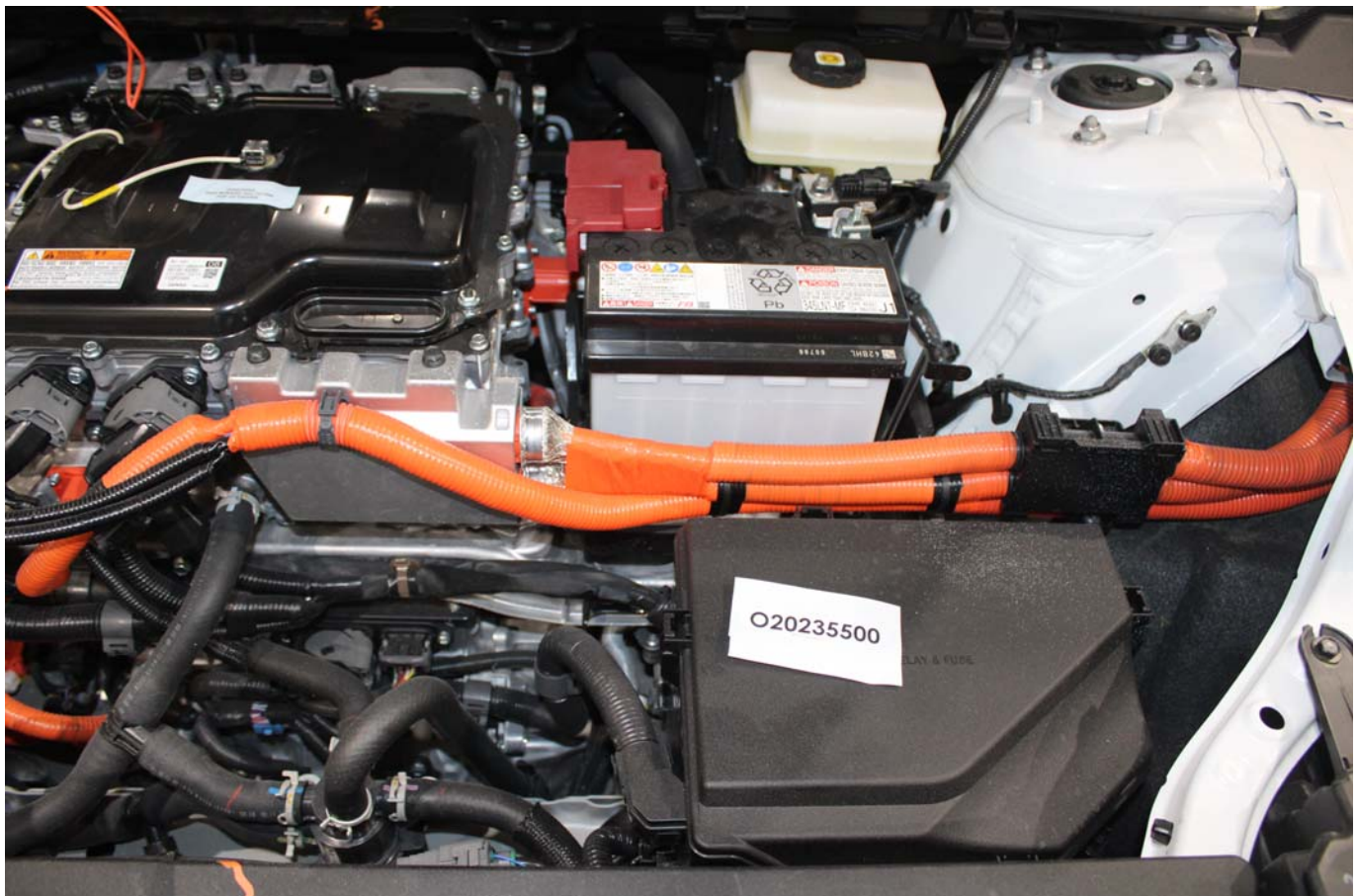
Photo No. 305-01 - Auxiliary Power Module Warning Label
