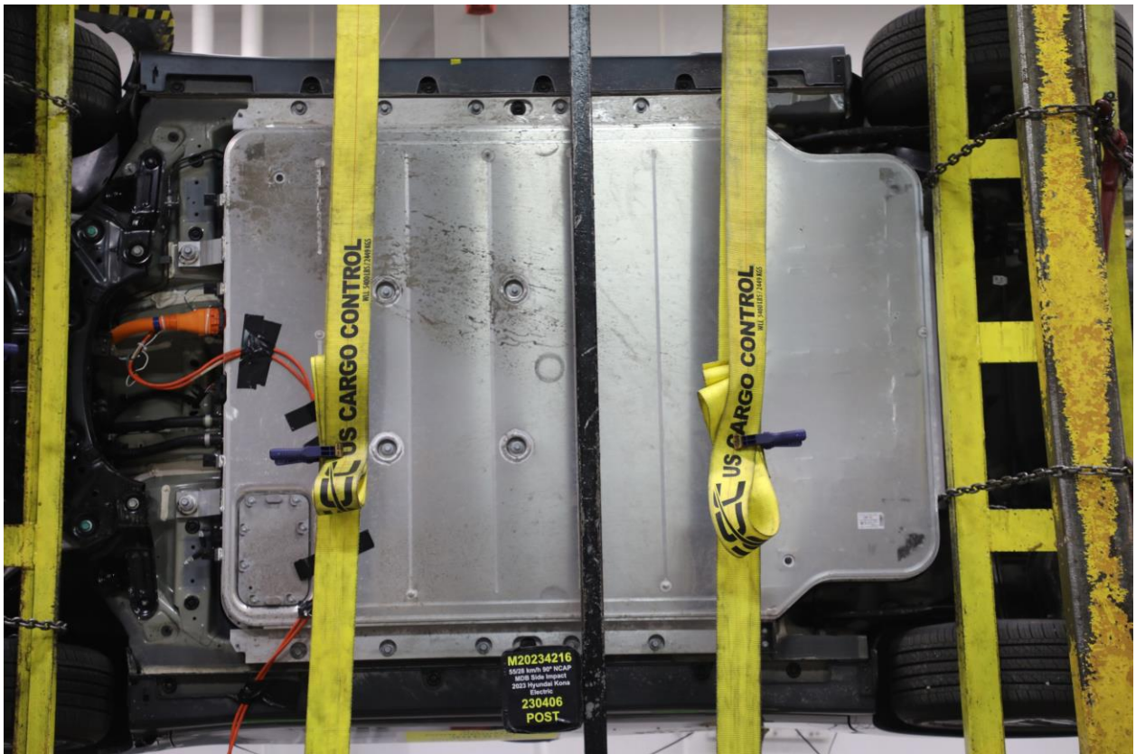
305-15 Post-Impact View of Propulsion Battery Module(s)
