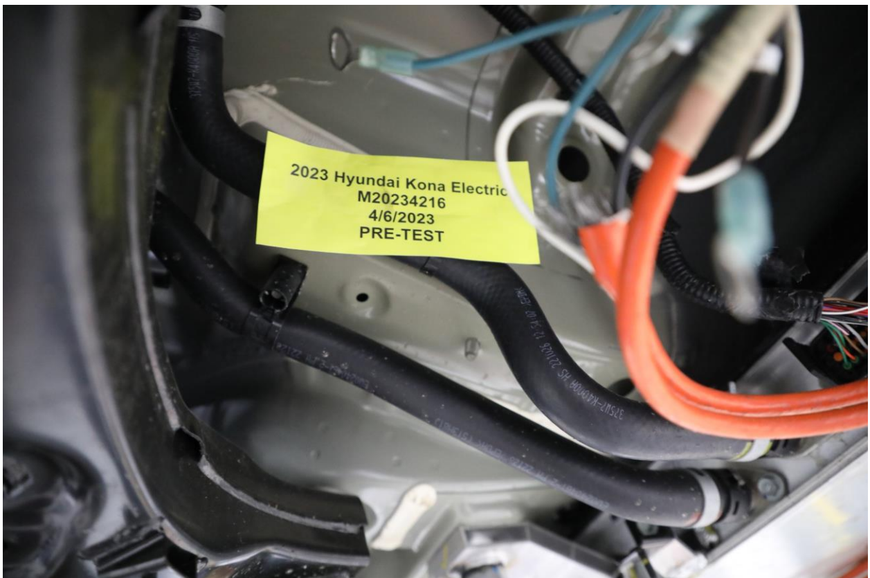
305-19 Pre-Impact View Propulsion Battery Venting System(s)
