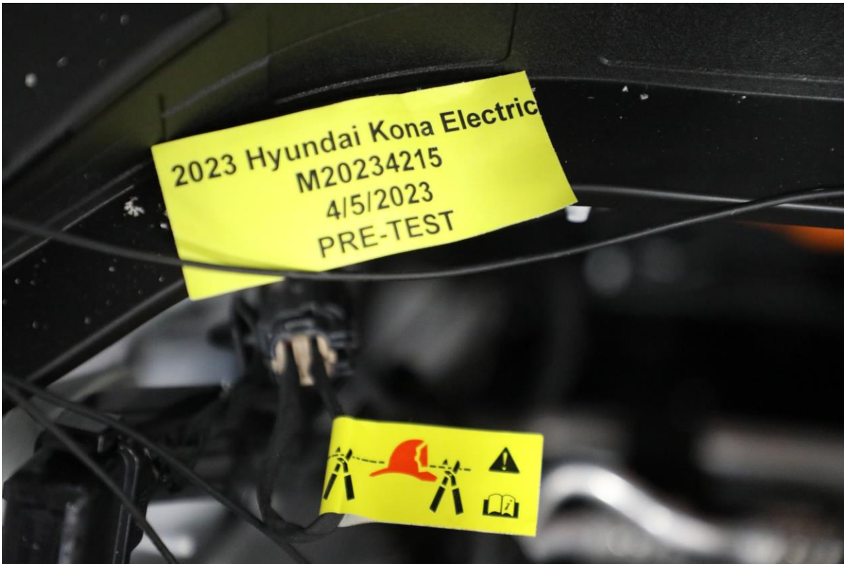
305-06 Manual High Voltage Service Disconnect in Place
