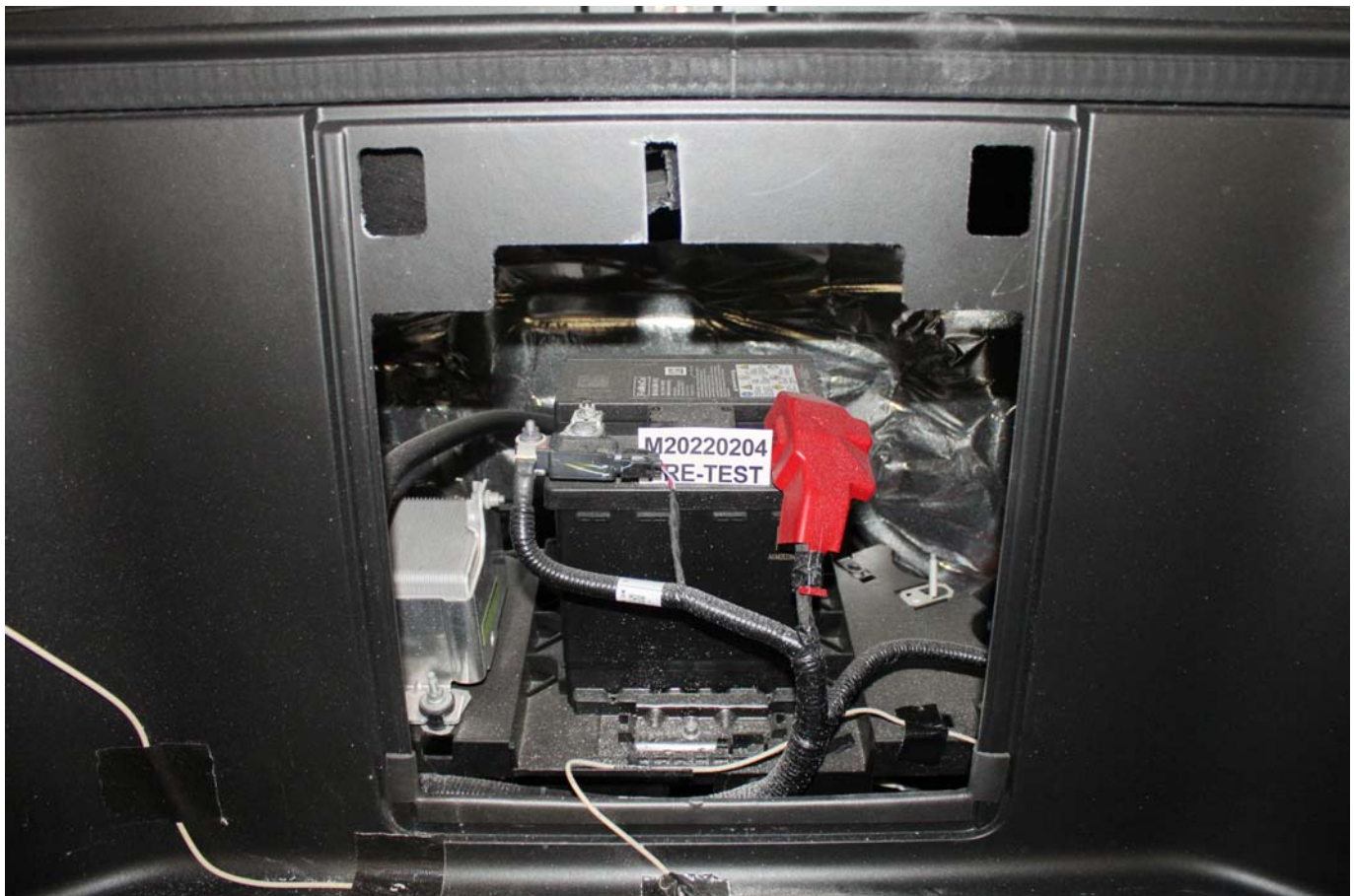
Photo No. 305-01 - Auxiliary Power Module Warning Label
