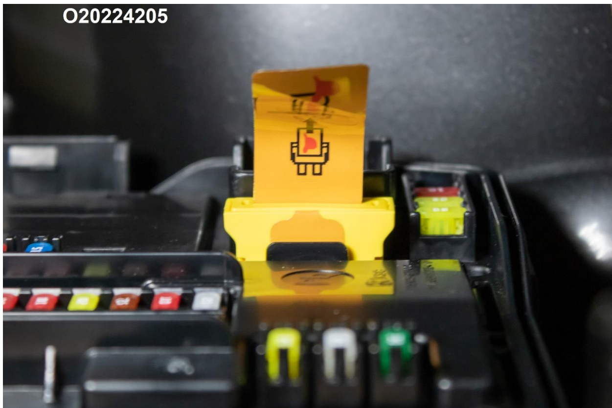
Figure 305-6: Manual High Voltage Service Disconnect in Place
