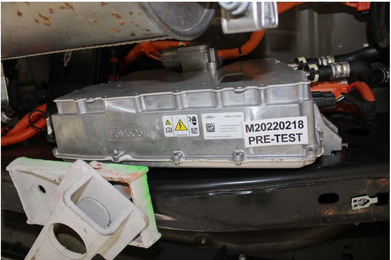
Photo No. 305-02 - Power Inverter Warning Label
