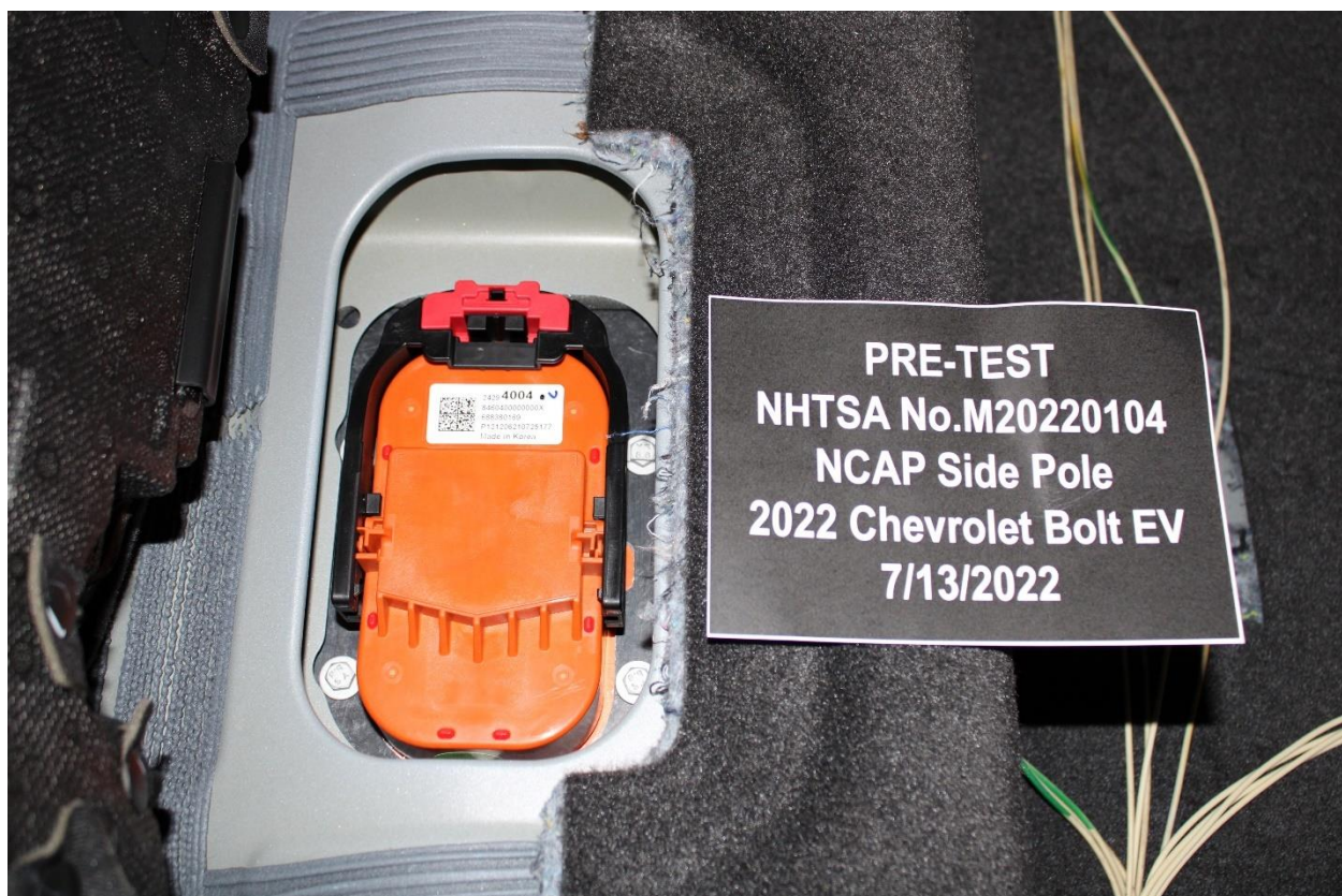
Figure 305-6: Manual High Voltage Service Disconnect in Place
