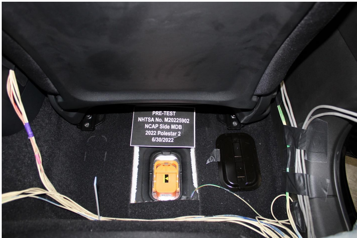
Figure 305-6: Manual High Voltage Service Disconnect in Place
