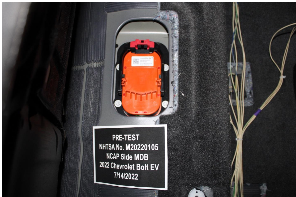
Figure 305-6: Manual High Voltage Service Disconnect in Place
