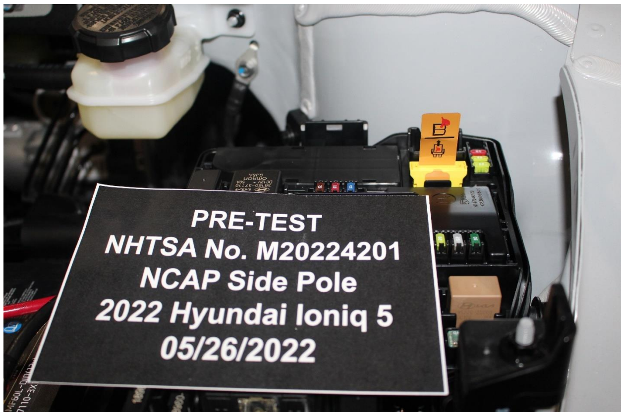
Figure 305-6: Manual High Voltage Service Disconnect in Place
