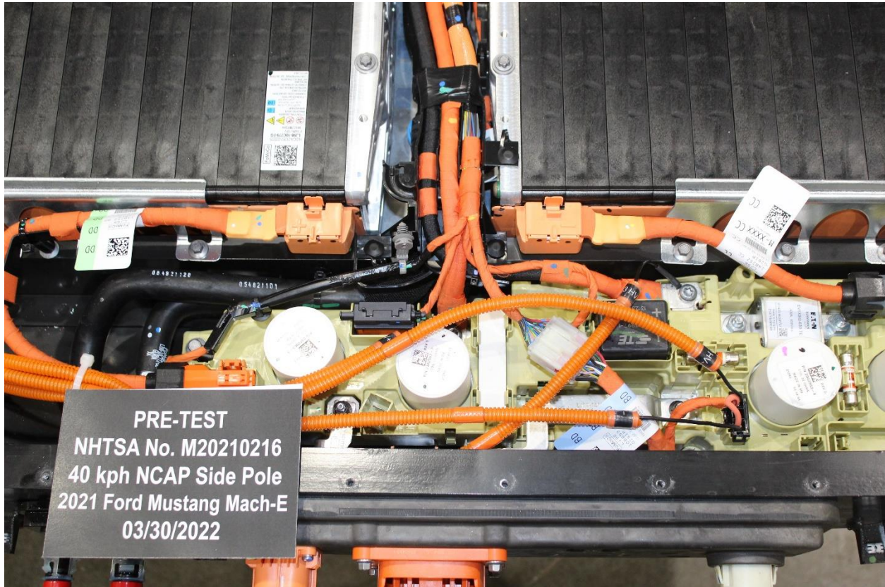
Figure 305-23: Pre-Impact Close Up View of High Voltage Leads Attached
