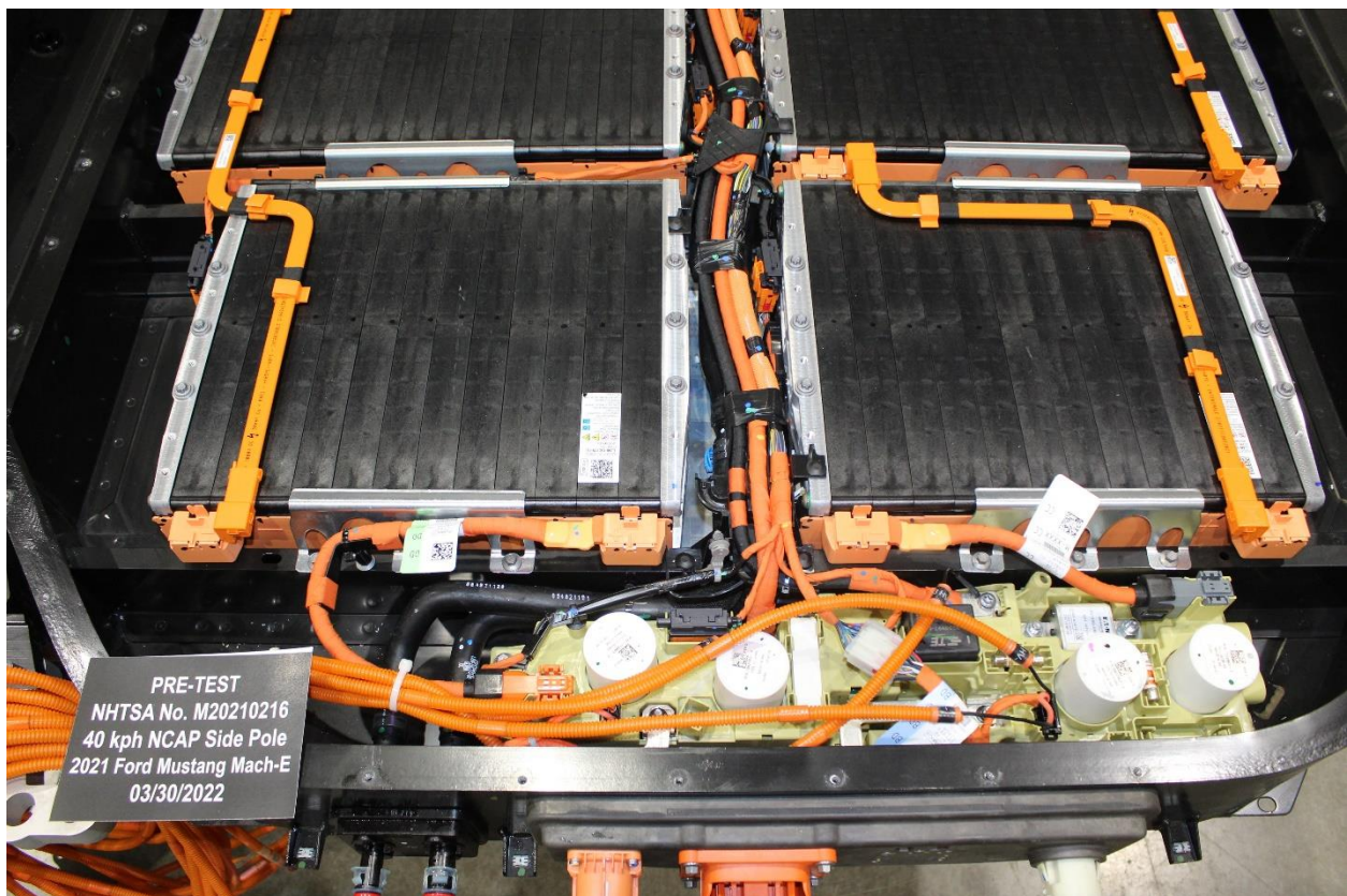
Figure 305-18: Pre-Impact View of High Voltage Interconnects
