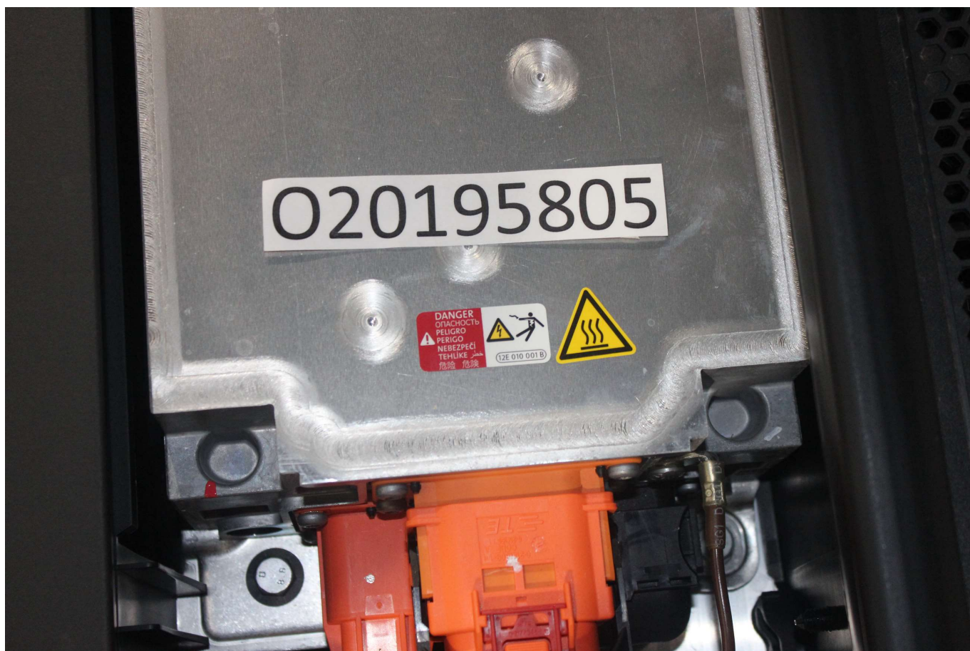
Photo No. 002 - Power Inverter Warning Label
