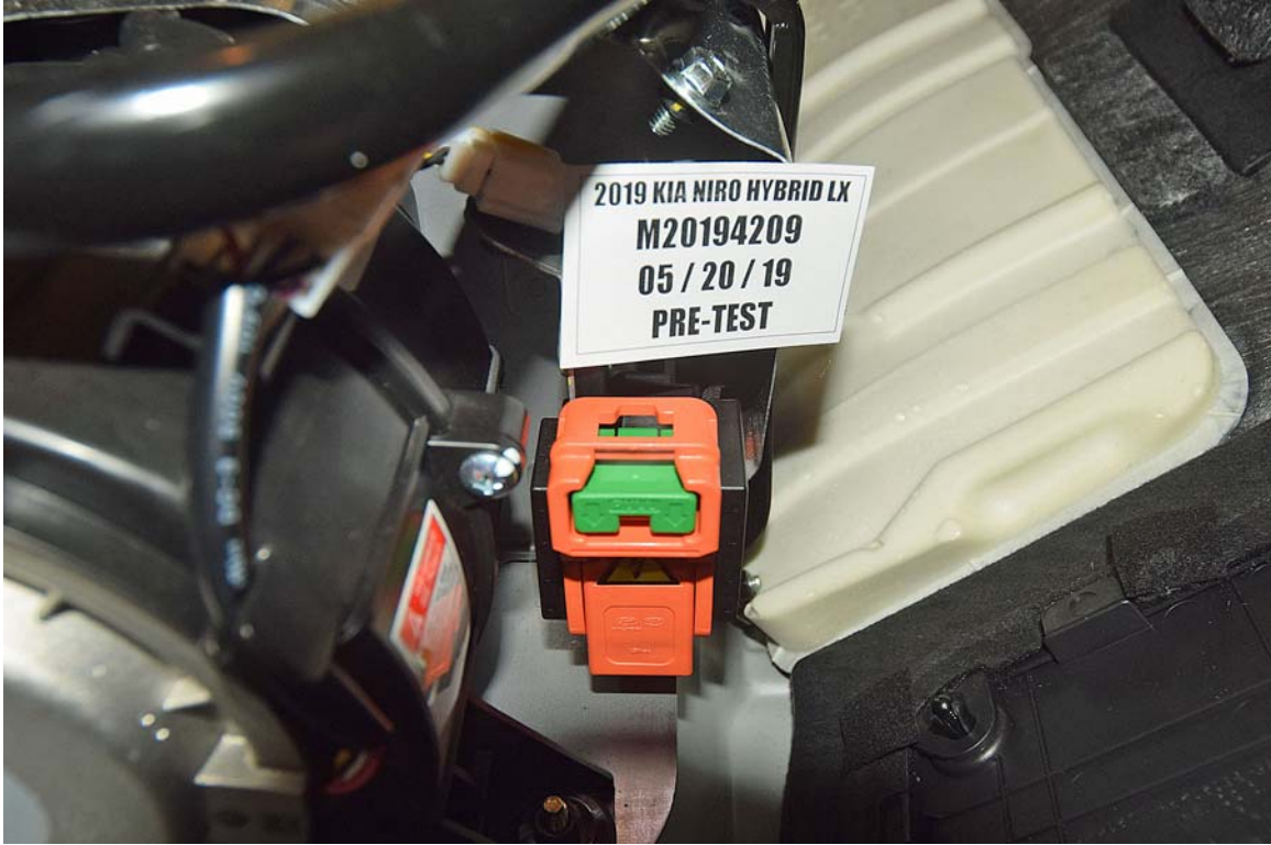
FIGURE 6. Manual High Voltage Service Disconnect in Place
