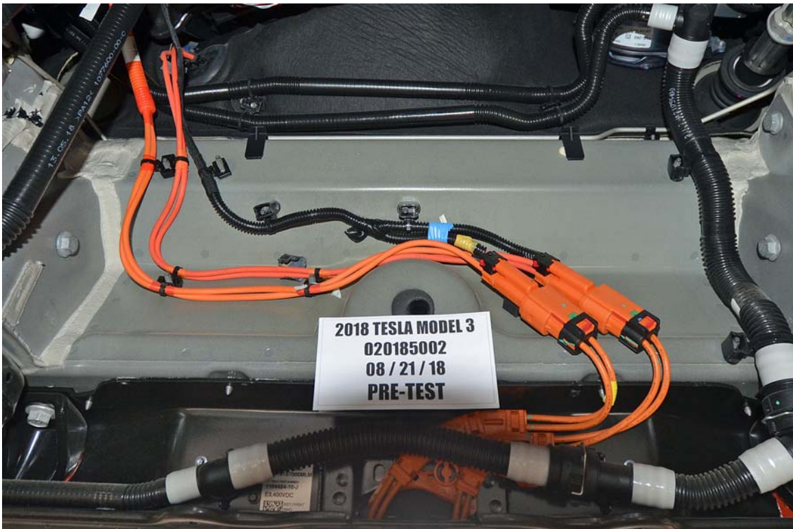
FIGURE 19a. Pre-Impact View of High Voltage Interconnect(s)
