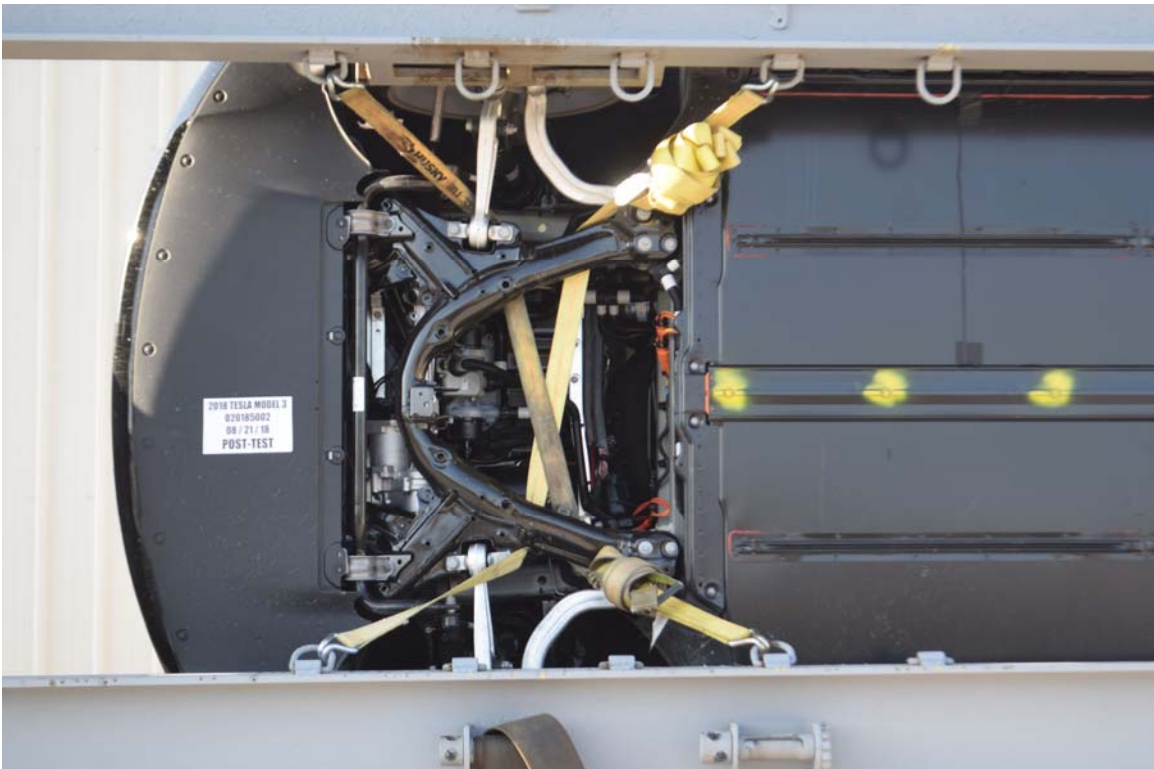
FIGURE 10. Post-Impact Front View of Propulsion Battery
