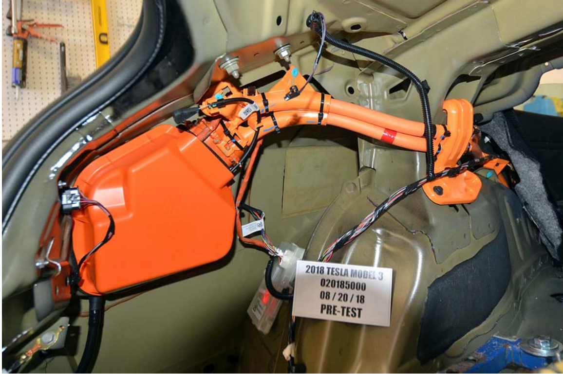
FIGURE 19a. Pre-Impact View of High Voltage Interconnect(s)
