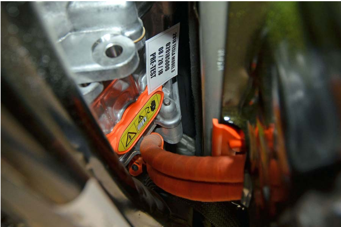
FIGURE 2b. Power Inverter Warning Label
