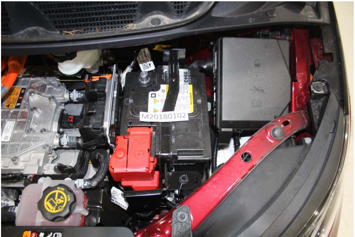
Photo No. 001 - Auxiliary Power Module Warning Label
