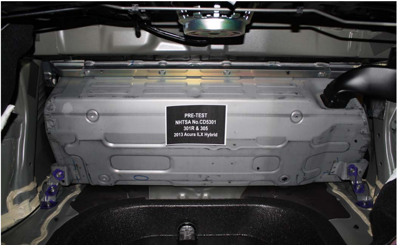
Figure A-49: Pre-Impact View of Propulsion Battery
