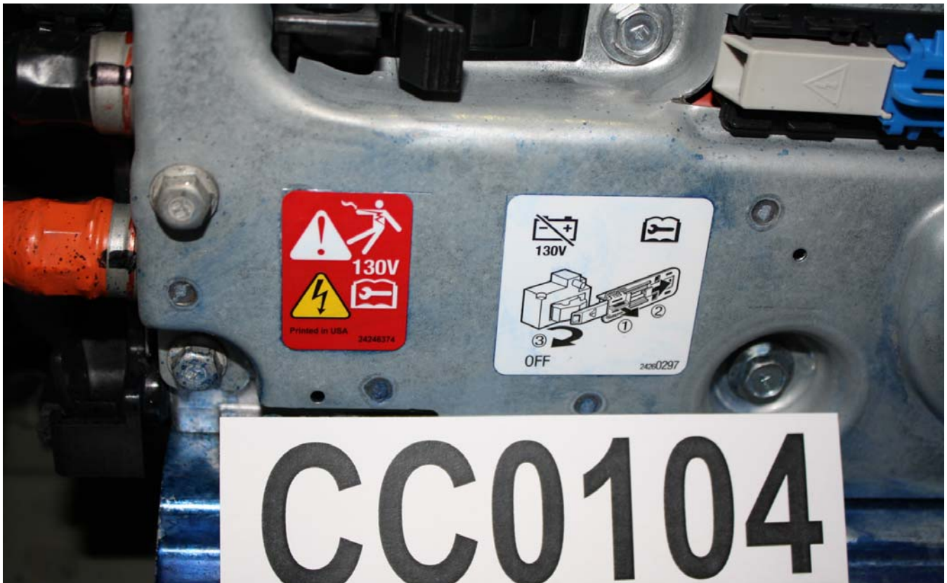
Figure A-42: Power Inverter Warning Label
