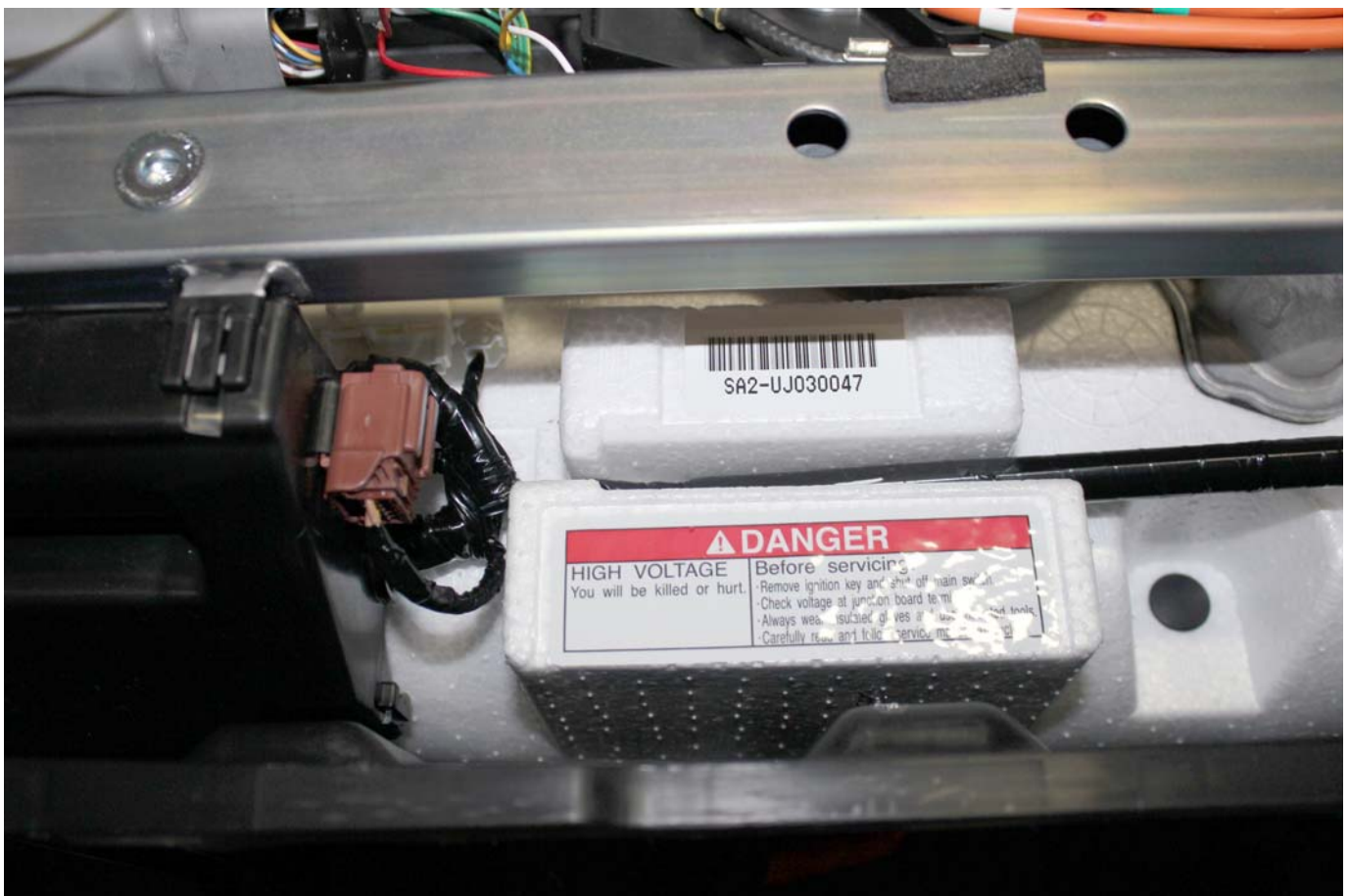
Labels and Markings
