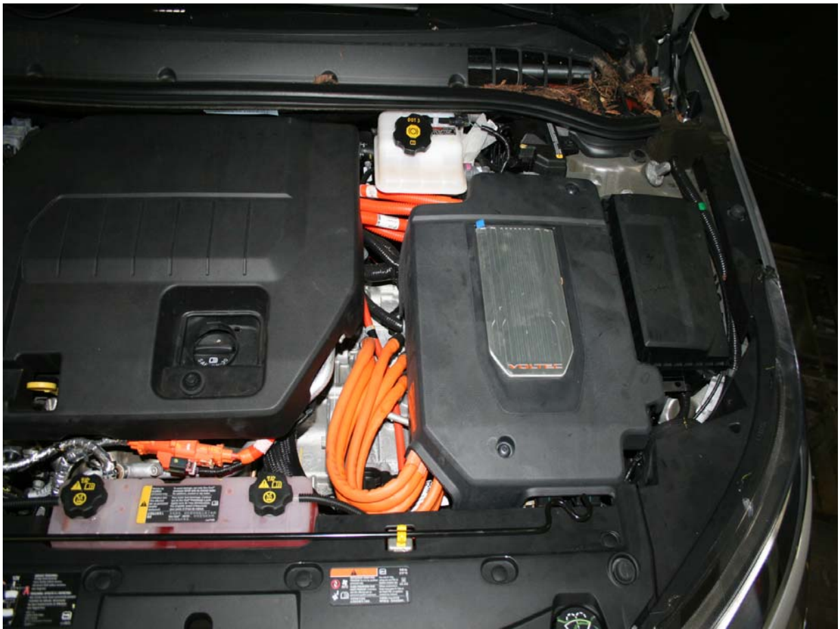
Power Inverter Warning Label/Location
