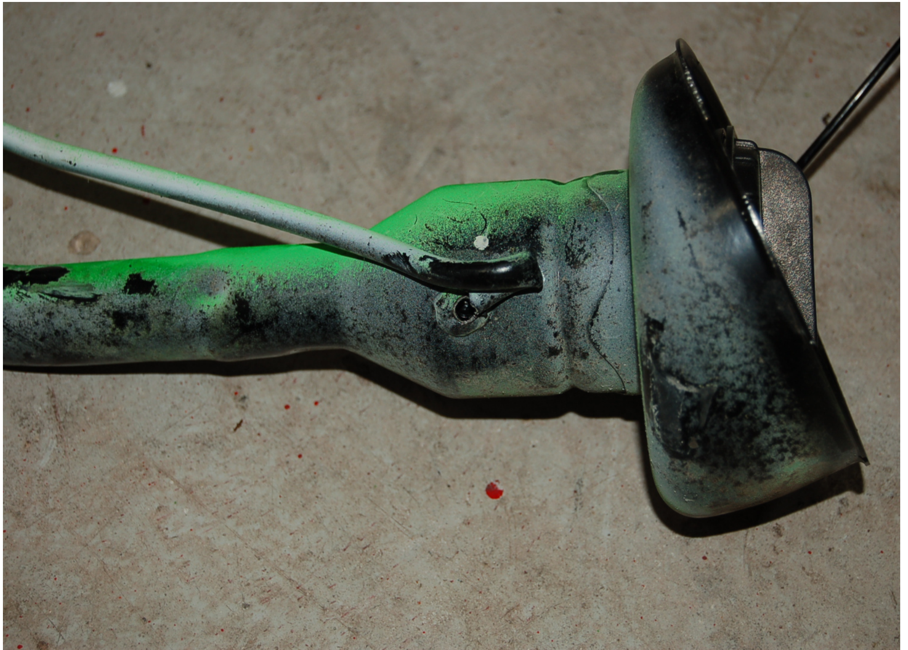
Leak Point at 0°
