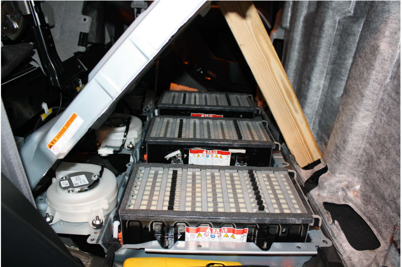
Figure A-33: Pre-Test Battery Propulsion Module(S) View
