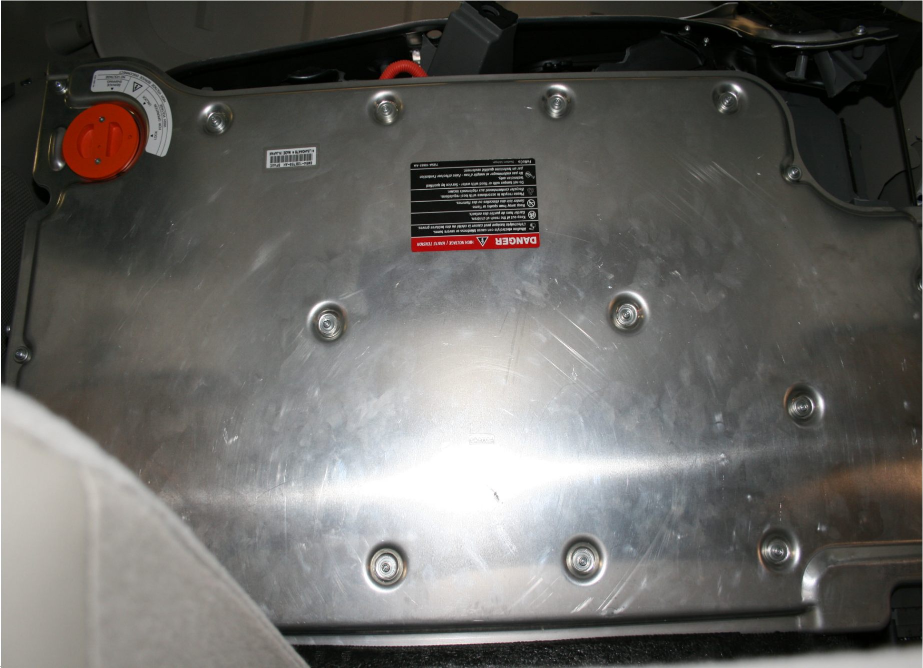
Post-Test Vehicle Pass. Compartment Adjacent to Propulsion Battery
