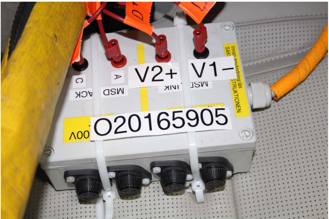
Photo No. 022 - Pre-Impact Close-Up View of High Voltage Leads Attached
