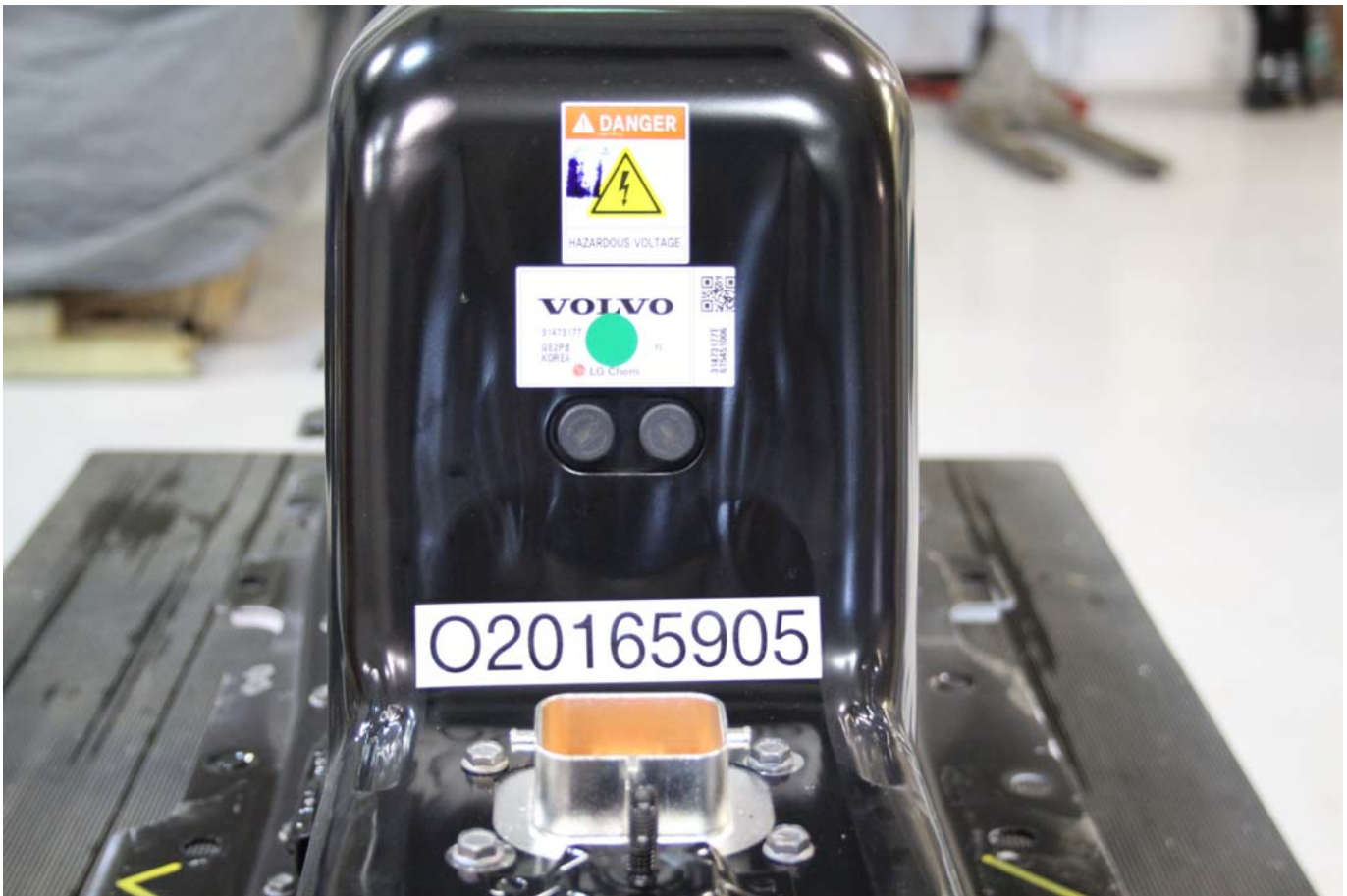
Photo No. 001 - Auxiliary Power Module Warning Label
