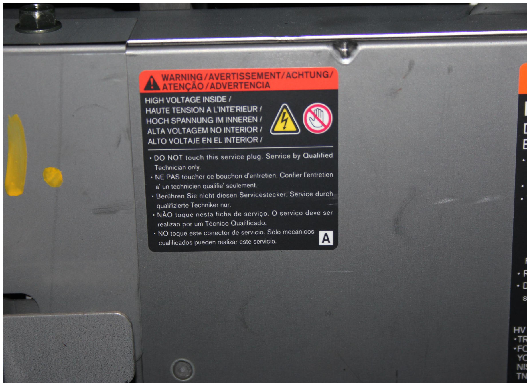
High Voltage Warning Label
