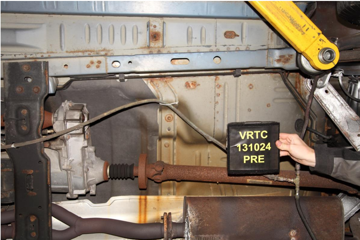
Figure A-23 Pre-Test Target Vehicle Fuel Line Close-up View
